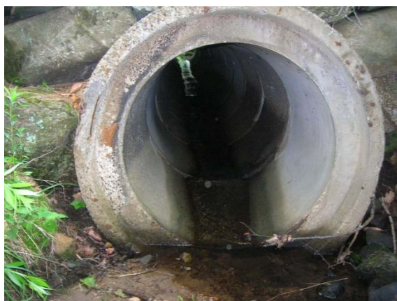
Figure 4. Inlet of undersized crossing on Reservoir Rd.
