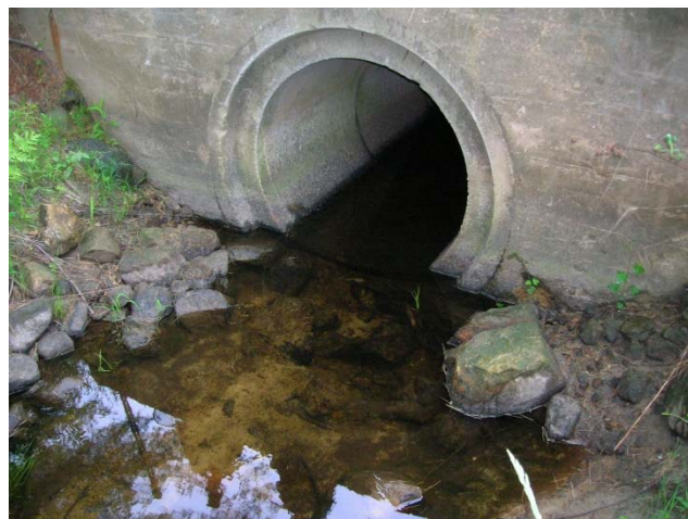
Figure 2. Undersized culvert crossing Winona Road
